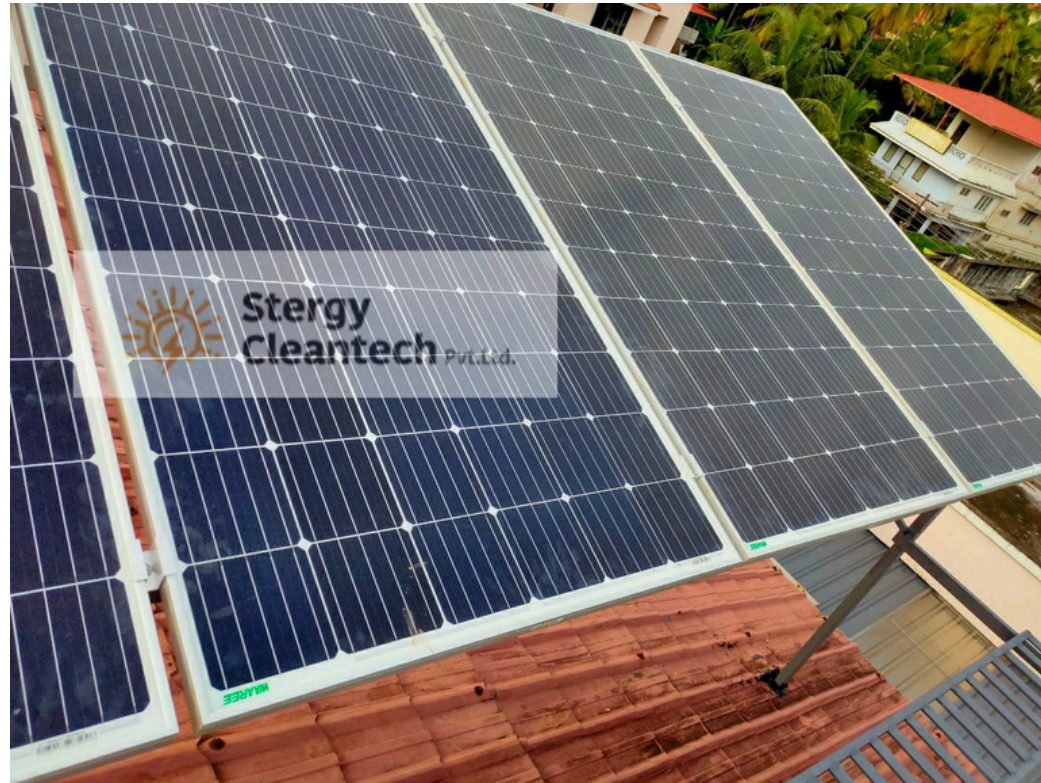
5 KW PROJECT SANAL KUMAR THRISSUR
